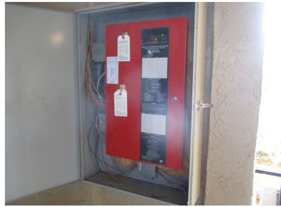
10 Fire Control Panel
