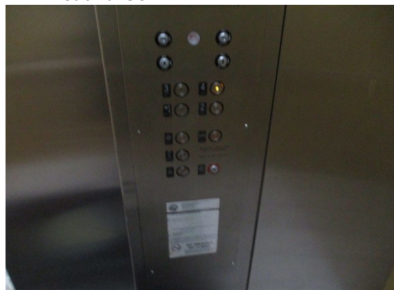
24 Elevator Cab Control Panel
