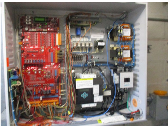
21 Elevator Control Board
