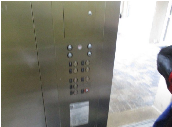
67 Elevator Cab Control Panel
